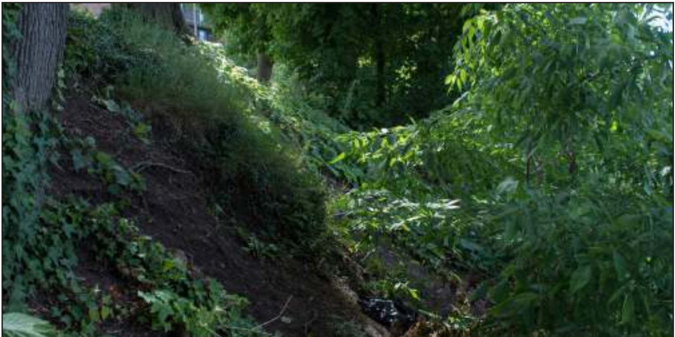
Bank erosion at Plaza Park
